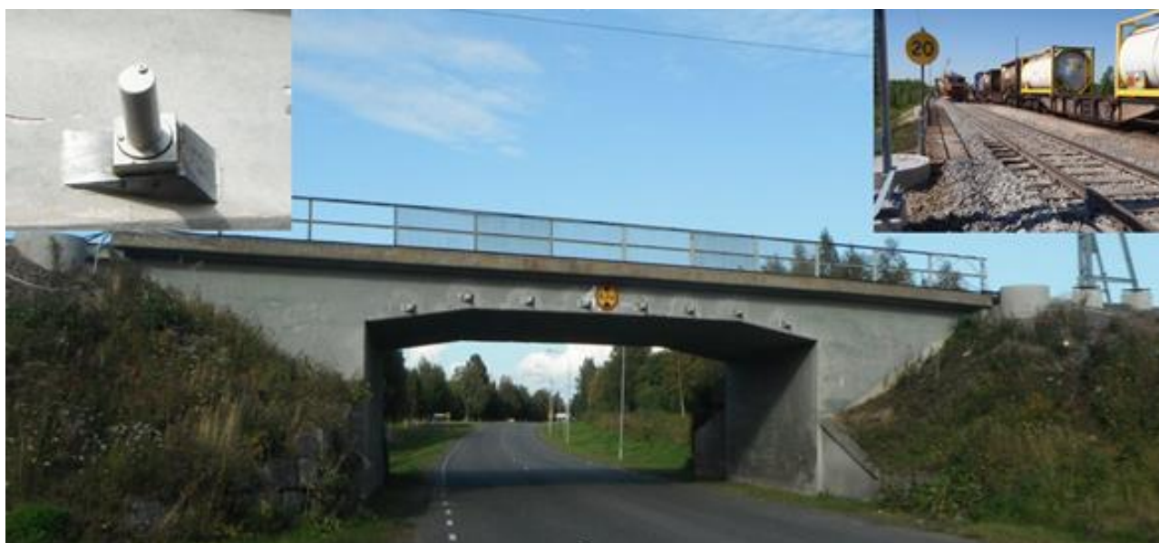
Figure 1. A concrete trough bridge strengthened with post-stressed bars installed in holes drilled through the slab (insert left). The two tracks on the top of bridge are also shown (insert right), Nilimaa [3]
