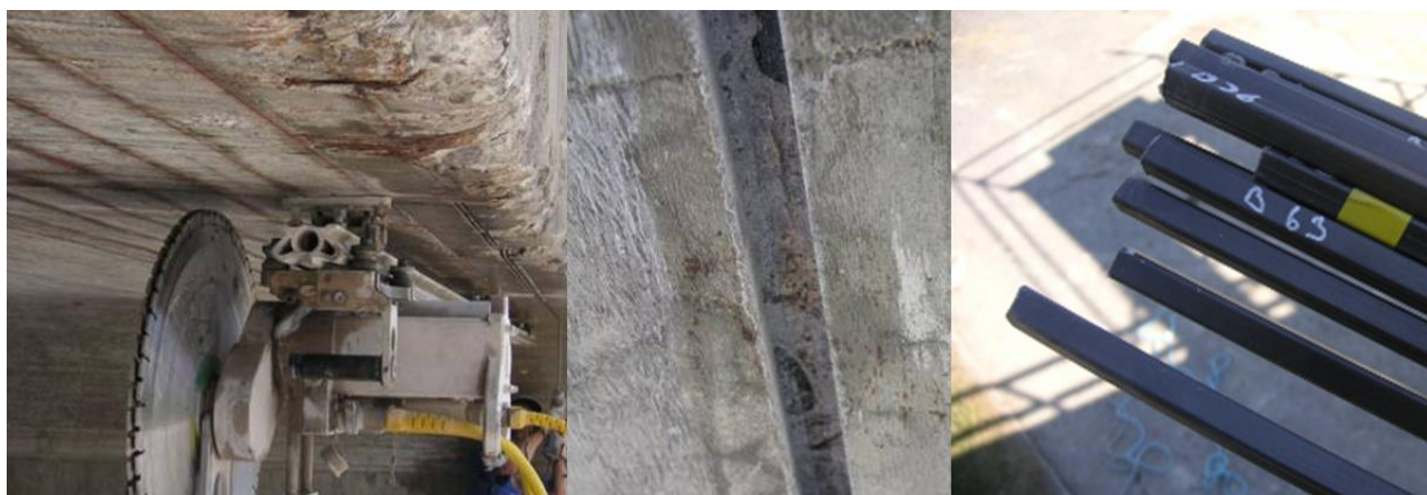
Figure 2. Near Surface Mounted Reinforcement (NSMR) are placed in groves grinded in the bottom of a slab (left, middle). Carbon Fibre Reinforced Polymer (CFRP) bars (right) can then be glued into the groves.
