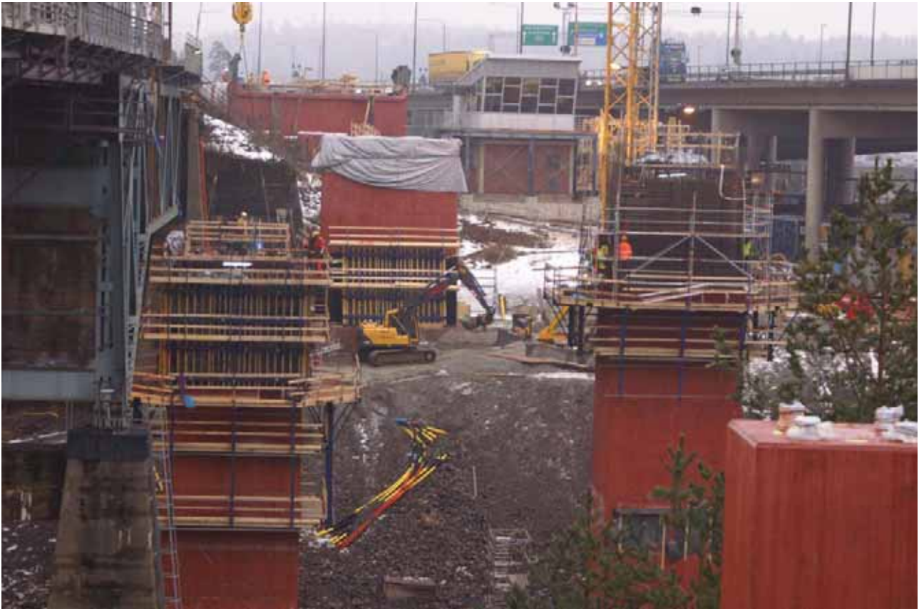
Figure 5. Structures with red concrete
