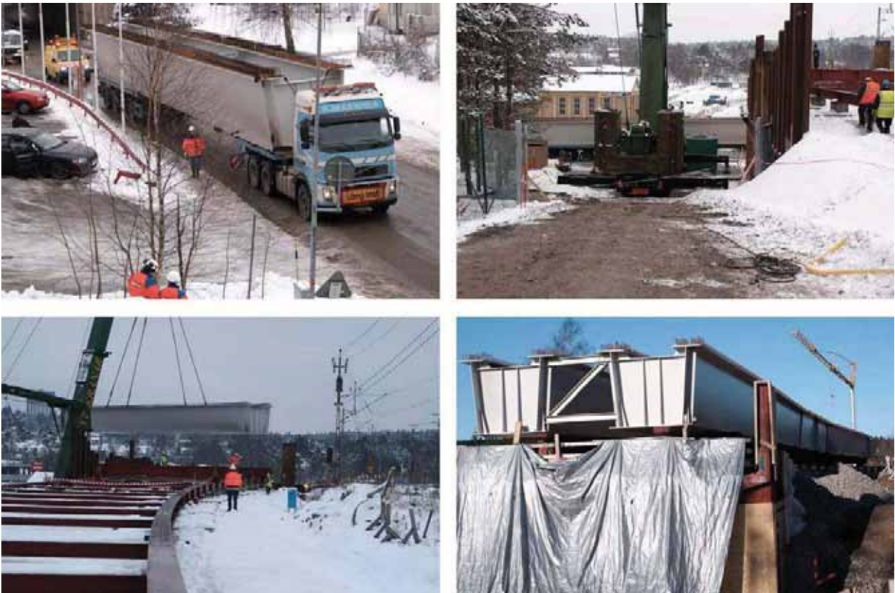
Figure 7. The arrival of the steel girders from Finland and the lifting operation from truck to launching track behind the abutment structure.
