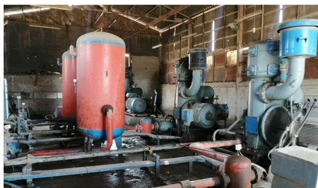
Figure 2. The main compressor house of the Qaleh-Zari Copper Mine.
