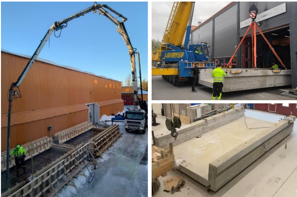
Figure 22. Casting Day for the two trough bridges (left), transportation of TB1 (right, top), TB1 inside the laboratory (right, bottom).
